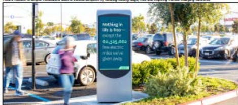
Above is a typical Volta installation showing one of our charging stations in a parking area.
